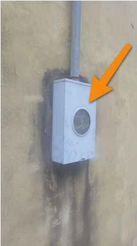
Meter pulled by the electric company
