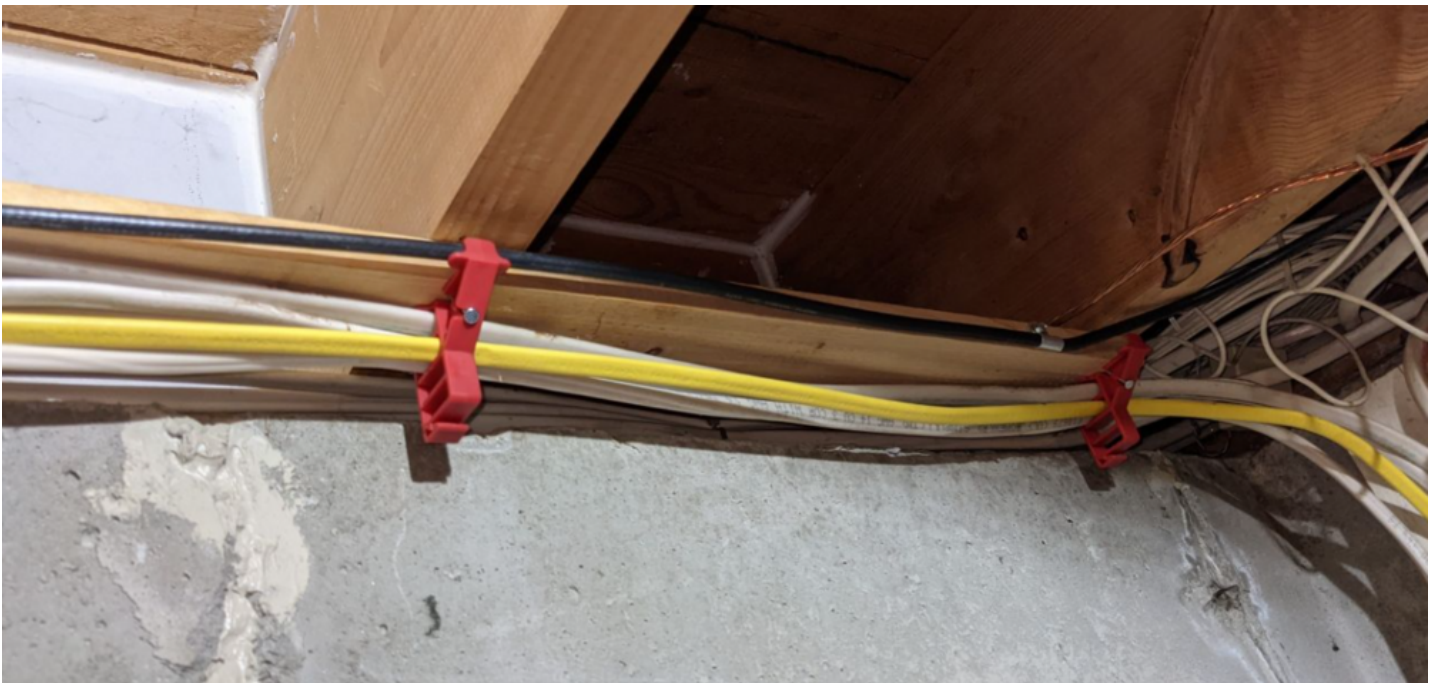
EXAMPLE ONLY: PROPERLY SECURED WIRES IN CRAWL SPACE FOR COMPARISON
