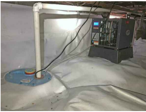
EXAMPLE ONLY (NOT INSPECTED HOME) SUMP PUMP AND DEHUMIDIFIER
