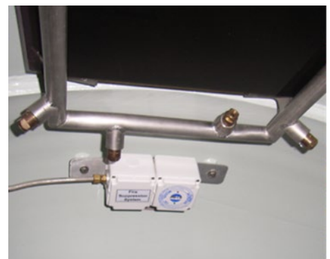
Overhead deluge nozzles
