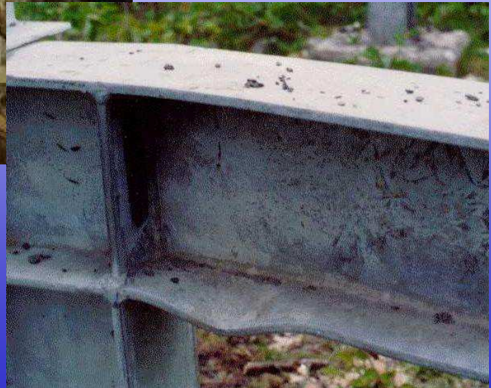
Local Buckling of the Beam Flange
