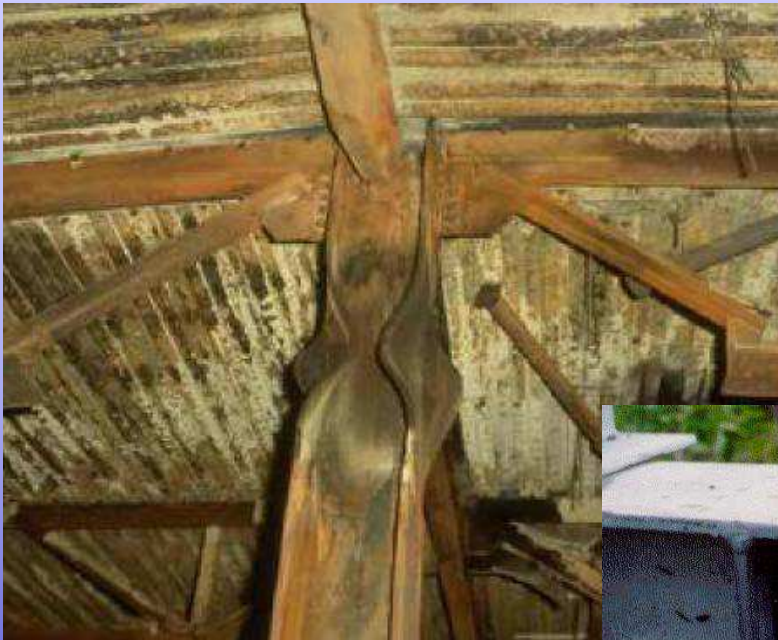
Local Buckling of the Column
