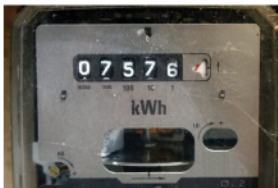
Figure 3 An electricity meter
