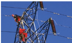
Figure 4 Engineers at work on the Grid. They certainly need a head for heights!
