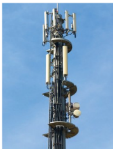
Figure 2 A mobile phone mast
