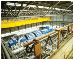
Figure 2 Inside a gas-fired power station
