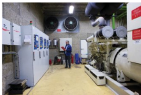
Figure 1 A standby generator
