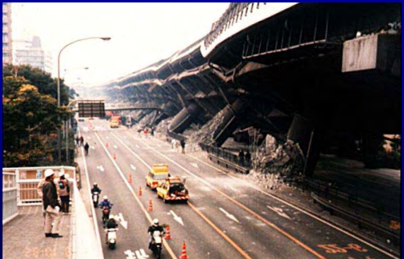
The Hanshin Expressway collapse was due to the very large horizontal components of the Hyogo-Ken Nambu earthquake of January 17, 1995 in Kobe, Japan.
