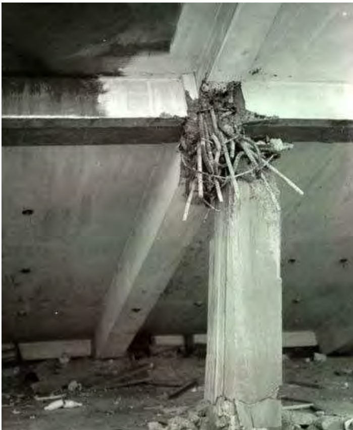
Detail of structural building failure caused by the earthquake in Cotabato, PHILIPPINE, August 16, 1976
