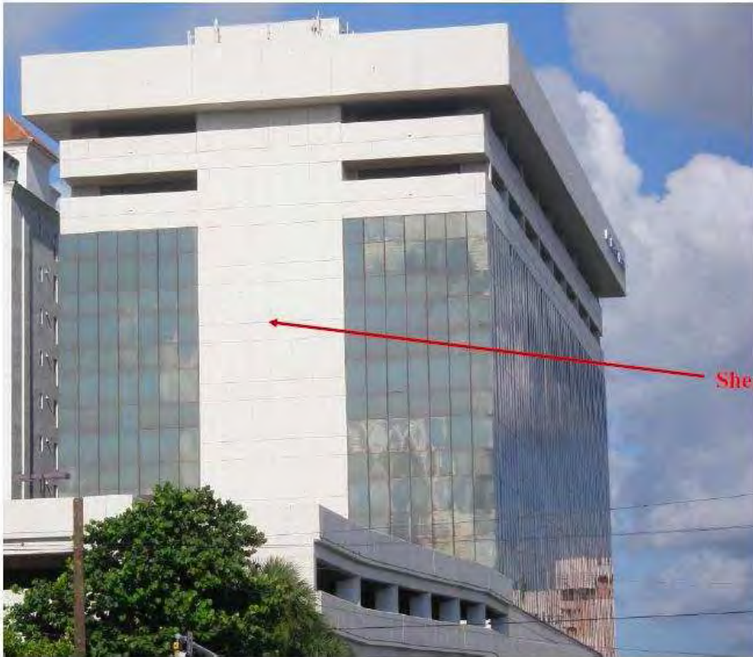
This lecture's problem is like this shear-wall at a building in Coral Gables (LeJeune and Valencia).
