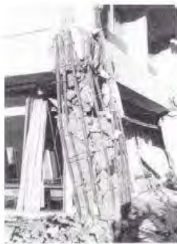
Brittle failure of a reinforced column
