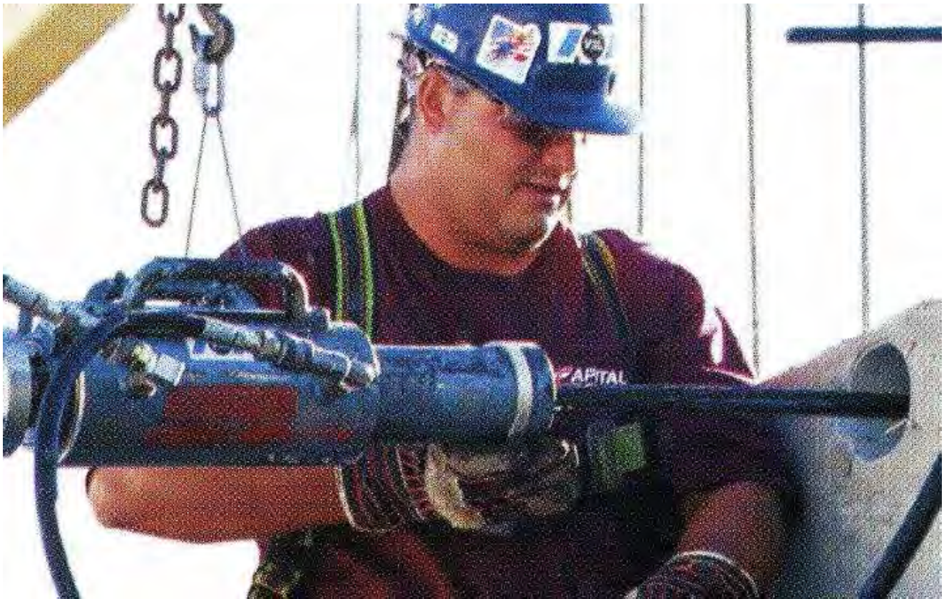
A heavy duty jack, used here to stress several tendons at the same location.
