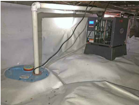
EAMPLE ONLY (NOT INSPECTED HOME) SUMP PUMP AND DEHUMIDIFIER
