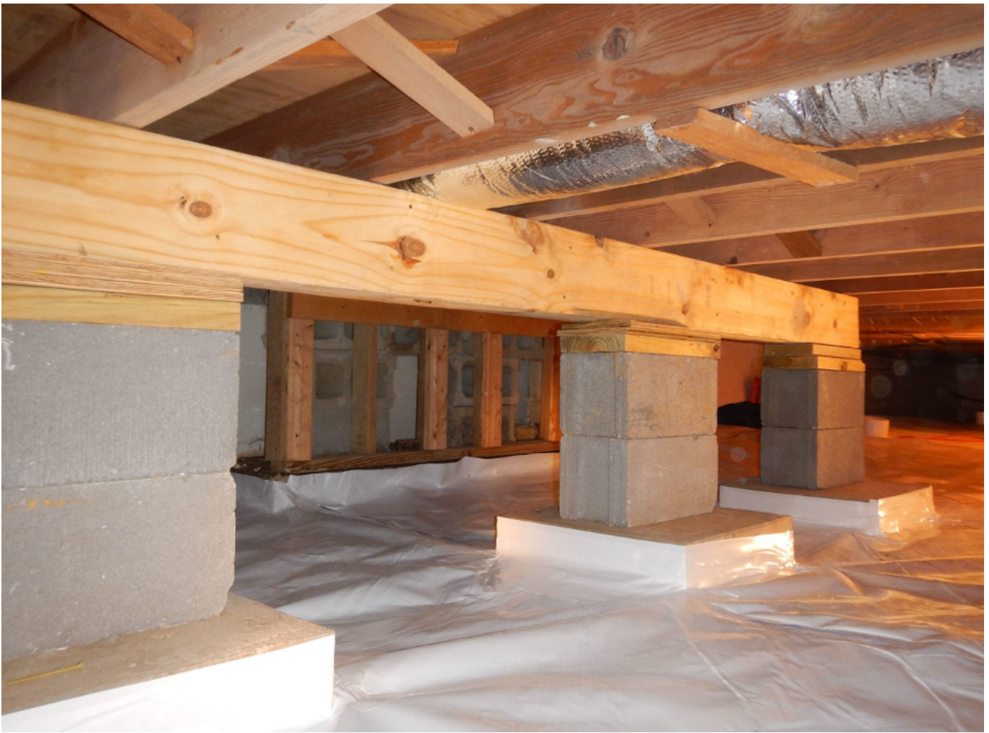
EXAMPLE OF ADDITIONAL PEIRS AND GIRDER BEAMS (CHEAPER OPTION WITH CONCRETE BLOCKS)
