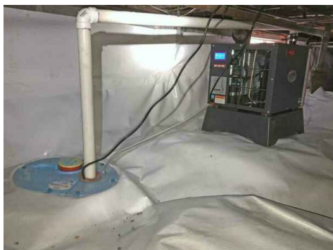
EXAMPLE ONLY (NOT INSPECTED HOME) SUMP PUMP AND DEHUMIDIFIER
