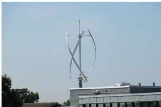
Figure 21 Microgeneration – a small wind turbine on the roof of a school
