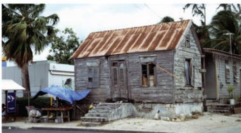
Figure 3 Poor-quality housing in Oisins, Barbados
