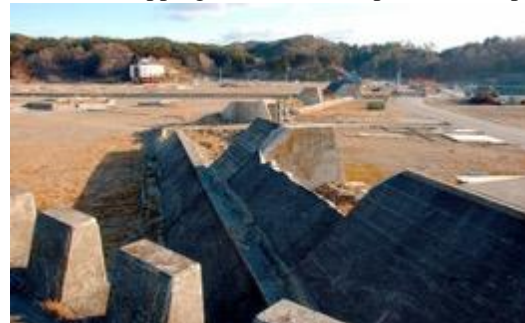
Fig.1 2011 Japan Earthquake tsunami Disaster area 561Km 2 .The Taro district where there was a large X-shaped seawall with a total length of 2.4 km and a sea-level height of 10 m. The seawall collapsed in an instant in a range of about 500 meters, killing nearly 200 people at 2011 Tsunami.
