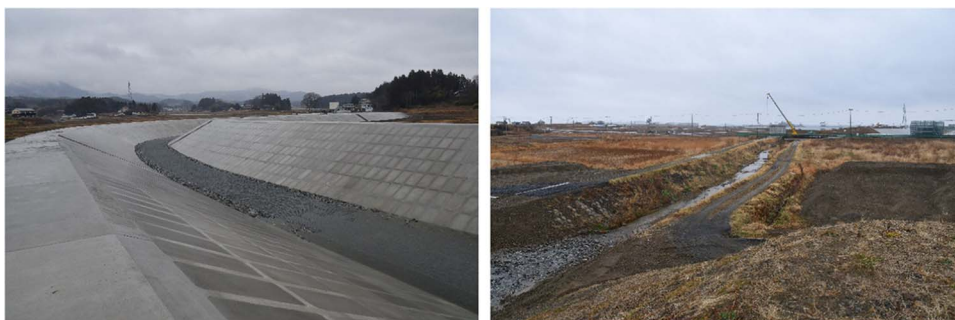
Fig. 5. Constructed section (left) and unconstructed section (right) at Okinota River in Miyagi prefecture (Photos taken by Naoya Furuta).
