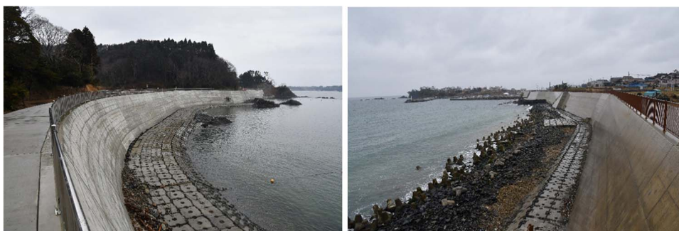
Fig. 4. Sea walls constructed just in front of the shorelines in Miyagi prefecture (Photos taken by Naoya Furuta).
