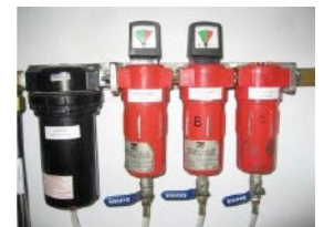
LP filtration system
