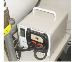
12 V DC transformer with ground-fault interrupter
