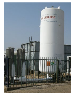
Cryogenic oxygen storage (LOX)
