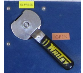
LP pressurization valve
