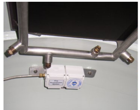
Overhead deluge nozzles
