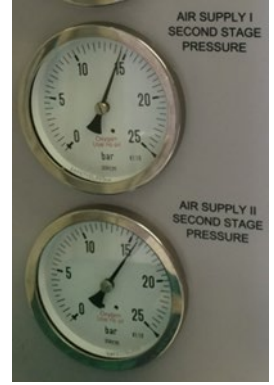
LP air supply pressure gauges
