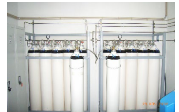
HP air cylinders
