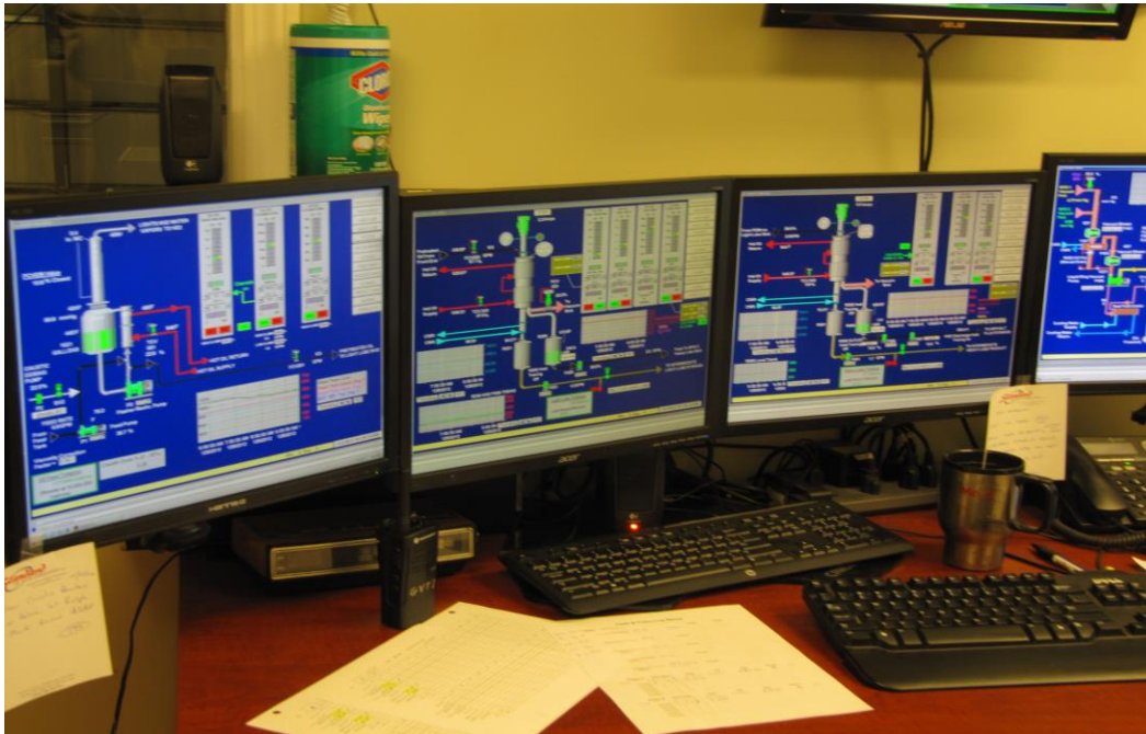
GVT Computer Control System
