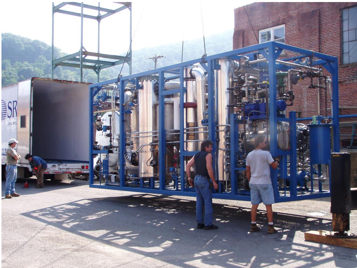
Solutions Recovery System Inc. Mobile Distillation Unit being installed
