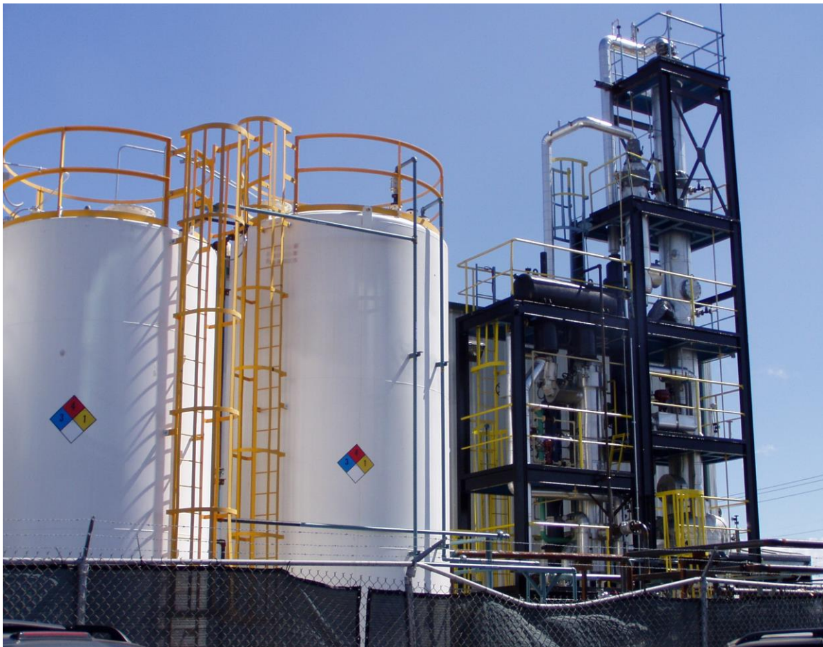
Tradebe Mixed Solvent Recovery System in operation
