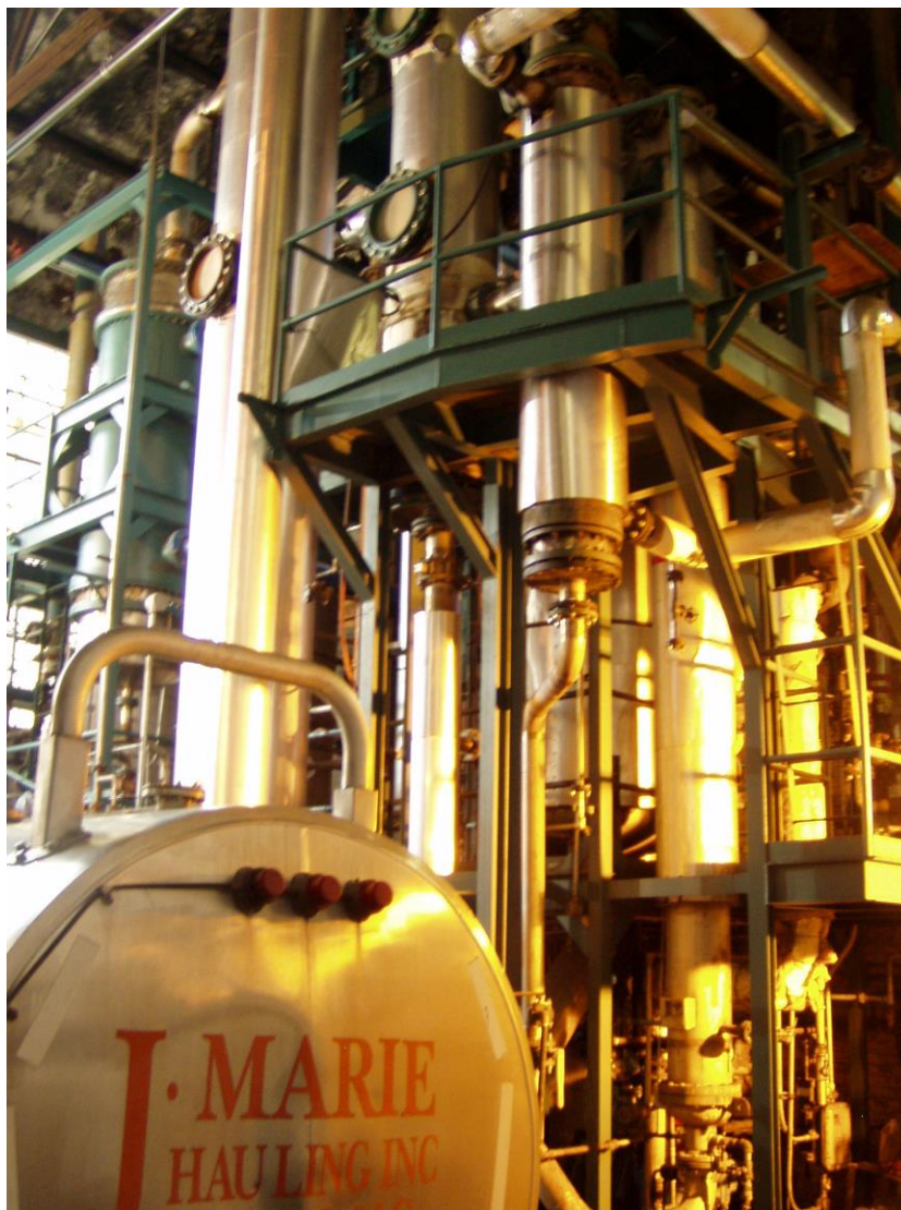
VEDCO LLC Glycol Recovery System
