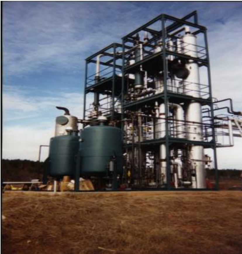
Sartomer Solvent Recovery System
